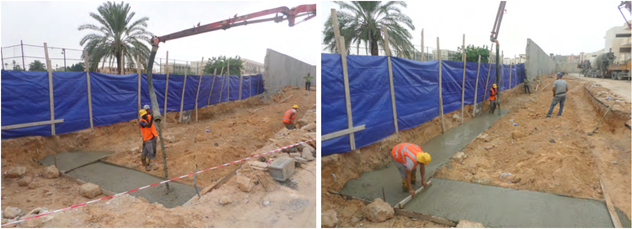
Construction works, HNEC new site, Sidi Al Masri, October 2018. Photo credits: Abdelhamid Kalai, UNDP, PEPOL.
