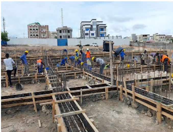
Mogadishu - construction of the NIEC data centre and warehouse is in progress and work is expected to be completed by the end of February 2020.
