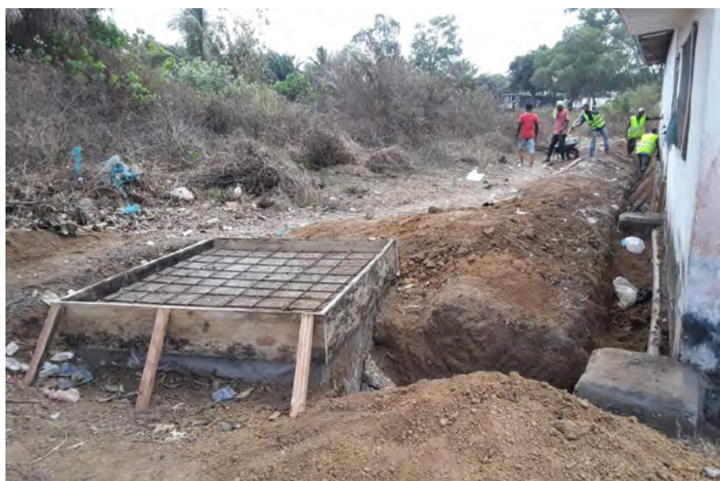
Renovation of Magisterial Warehouses of the National Election Commission in Progress in Buchanan. Photo credits: National Elections Commission of Liberia.
