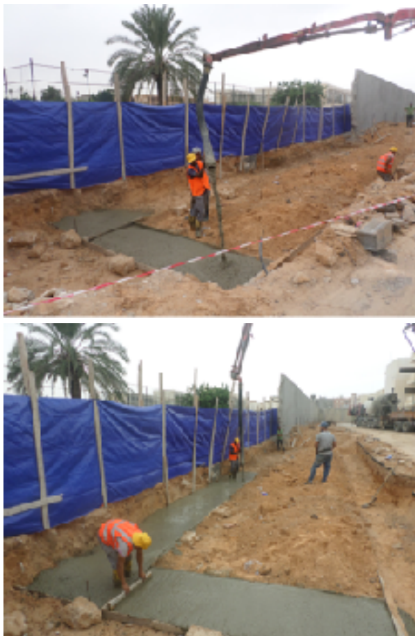
Construction works, HNEC new HQ site, Sidi Al Masri, October 2018. Photo credits, Abdelhamid Kalai, © UNDP.
